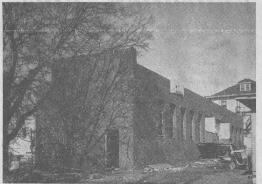
Construction of the second floor has begun on Bud Robinson Hall, formerly called the Cafeteria. This floor of the new facility will serve as a dormitory.
