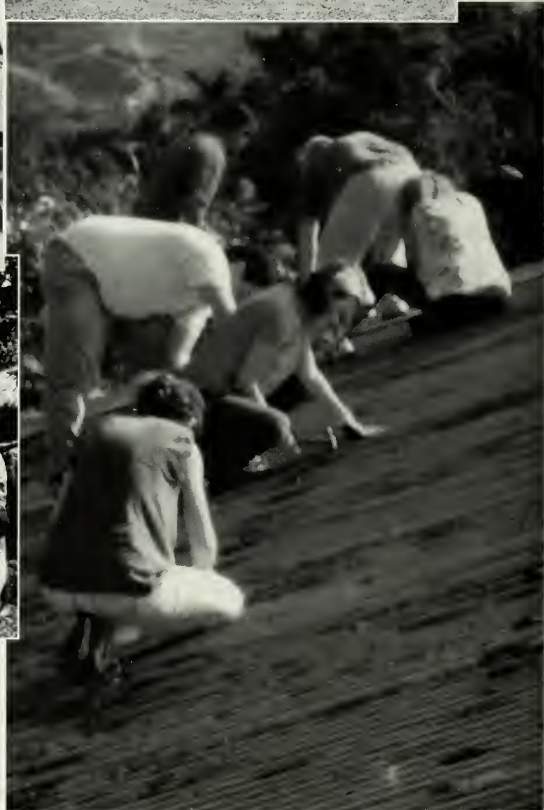
Students from the other Nazarene colleges and universities joined together to work on C.A.U.S.E. trips. The Puerto Rico team worked hard in the heat of the day replacing a rusty roof.
